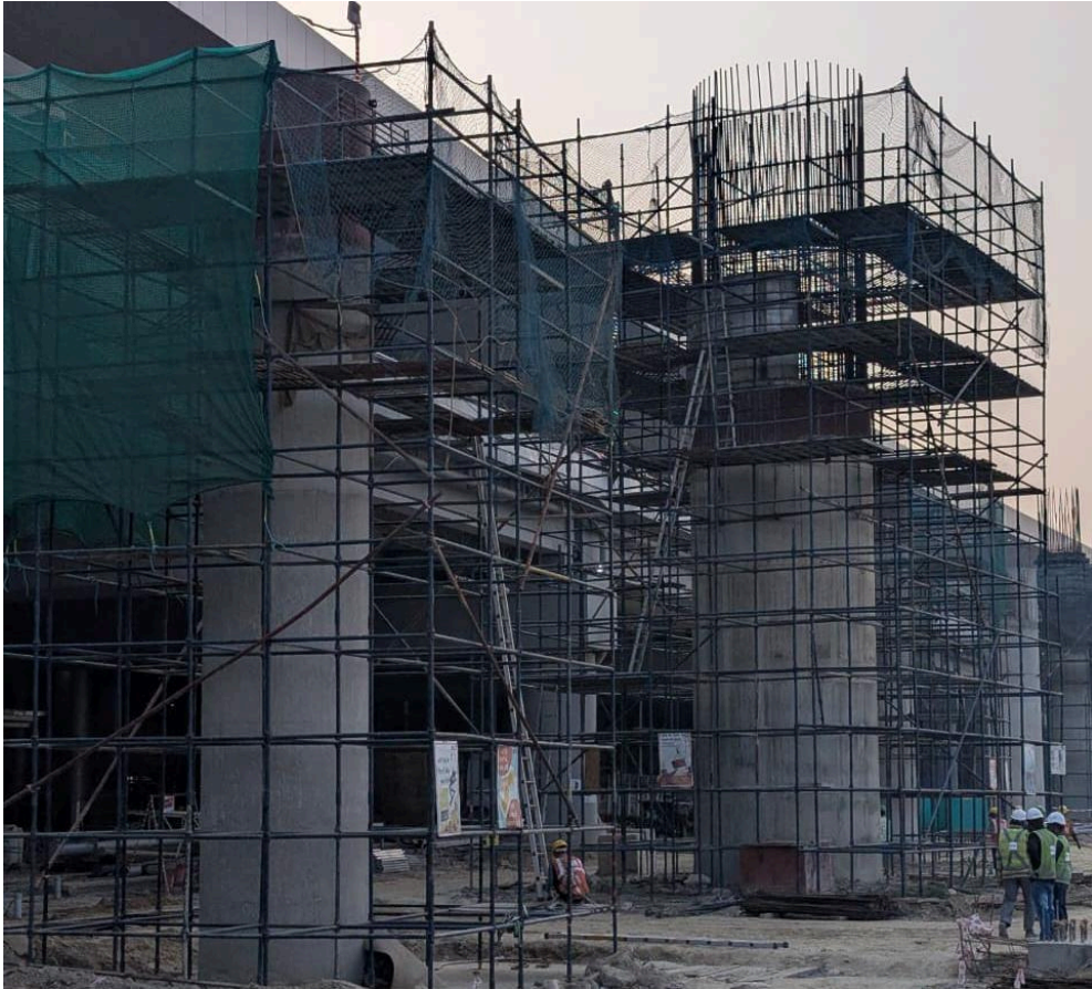
Phase 3 Canopy and Stack columns, construction ongoing. Structure work pending, Upon completion primary steel will be installed , MEP services will be completed which will make way for GFRP installation.
